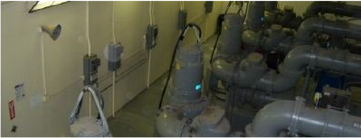
The mixed liquor pumps return flow to the bio selectors from the aeration basins, at a rate of 100% (but have the capacity for up to 500%).
