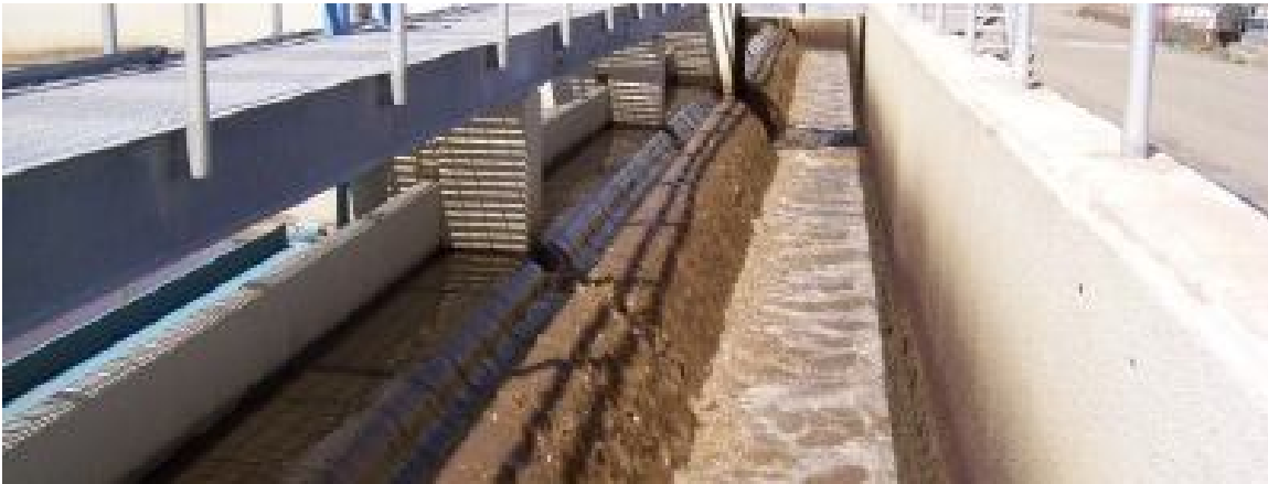
The Bio-selector Effluent flows to the aeration basins.
